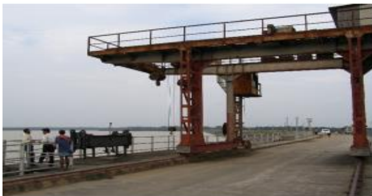
Distressed gantry crane
