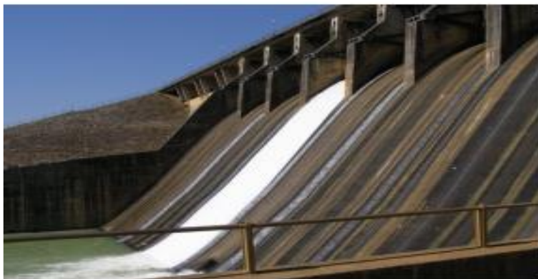
Leakage through control structure
