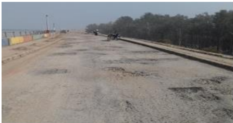
Poor condition of the dam top road
