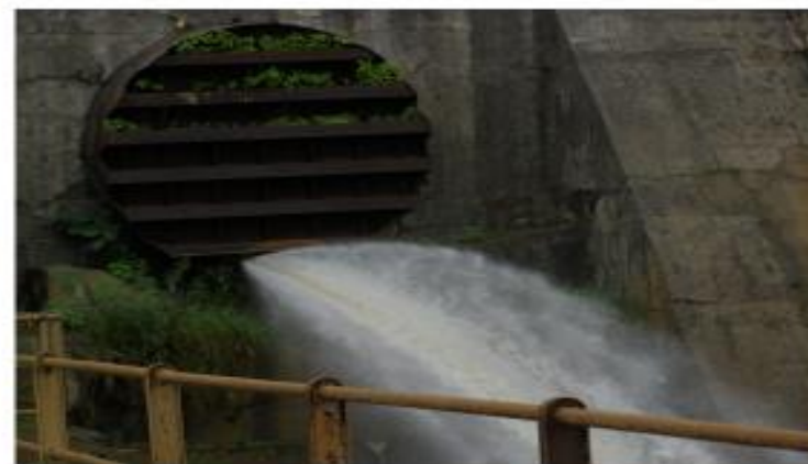
Leakage through penstock
