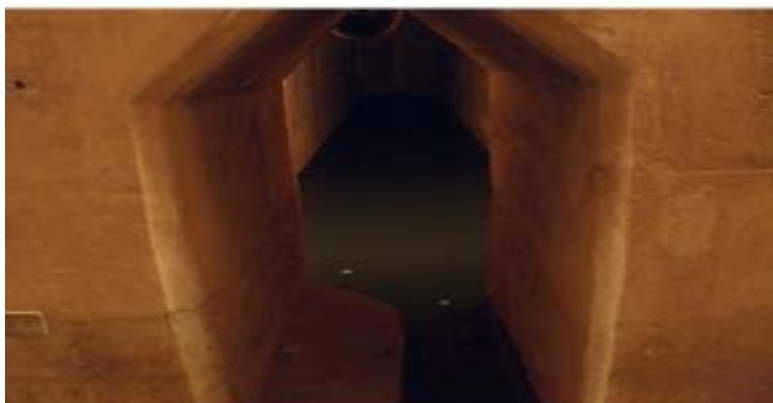
Crack in drainage gallery
