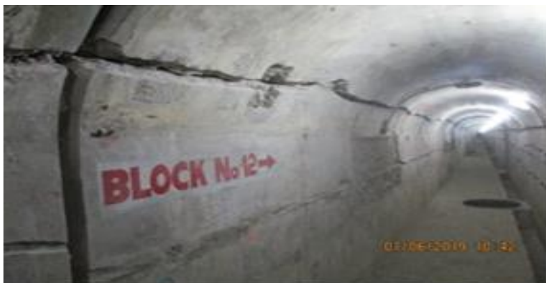
groove cut along the crack in gallery
