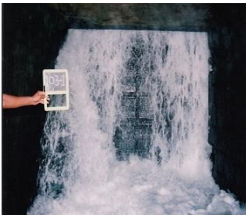
Leakages in +103' Level Sluice Gates before Rehabilitation (from KRS Dam site erection)
