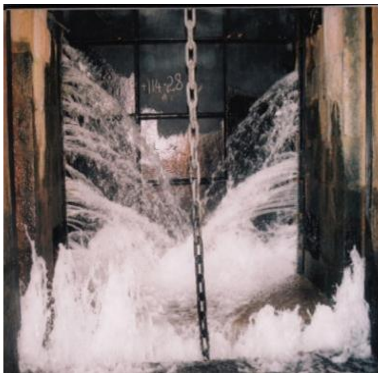
Leakages in +114' Level Sluice Gates before Rehabilitation (from KRS Dam site erection)
