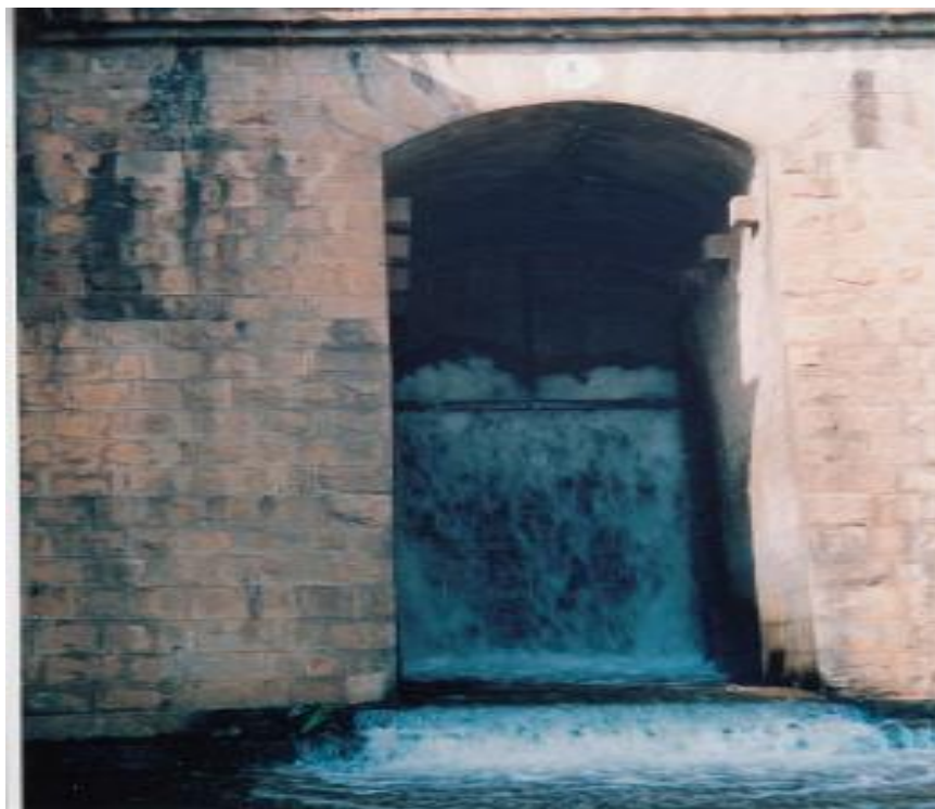
Leakages in +106' Level Sluice Gates before Rehabilitation (from KRS Dam site erection)
