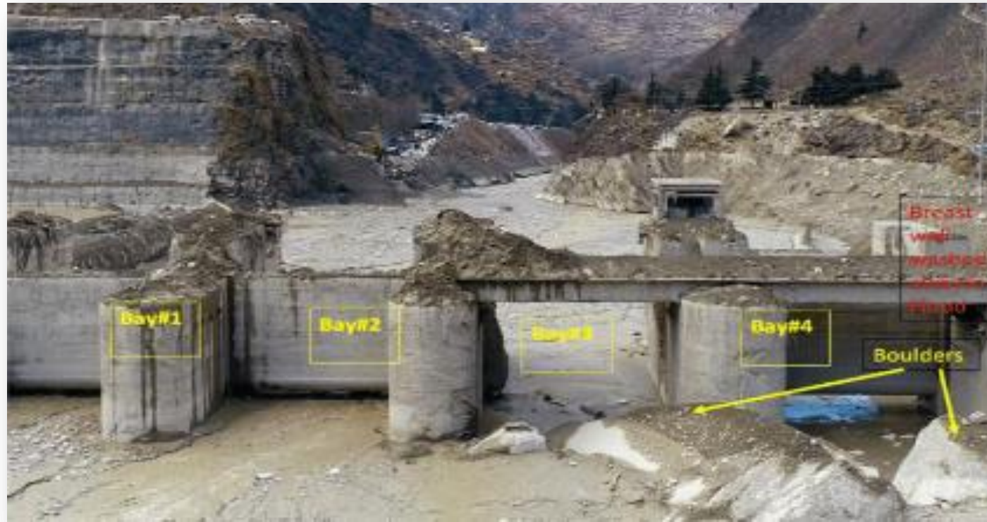
Damaged barrage of Tapovan HEP
