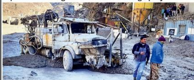
Locals inspect the site near damaged Dhauliganga hydropower project at Reni village, on Sunday
