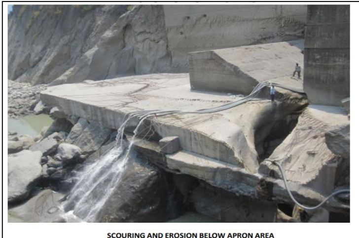
SCOURING AND EROSION BELOW APRON AREA
