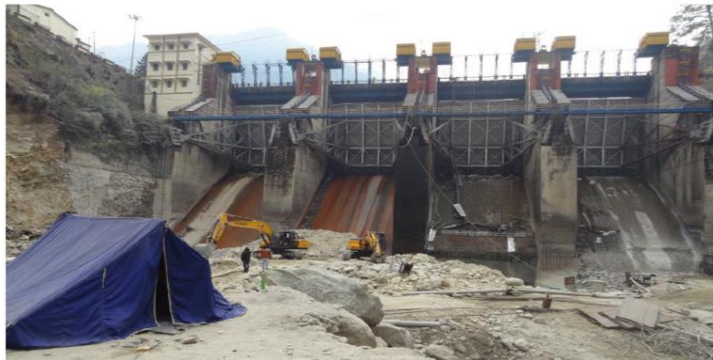
Repair of spillway glaciis and energy dissipator with M90 concrete (Maneri Dam, UJVNL).
