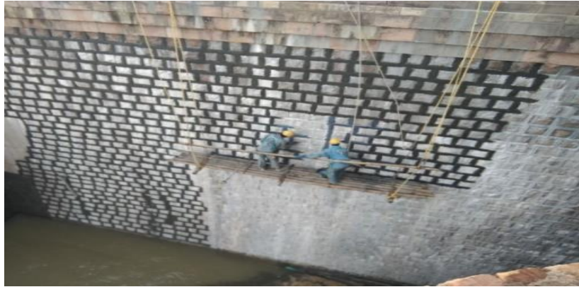
Racking & pointing of upstream face with UV resistant, high strength crystalline technology including underwater (Malaprabha dam, KaWRD).
