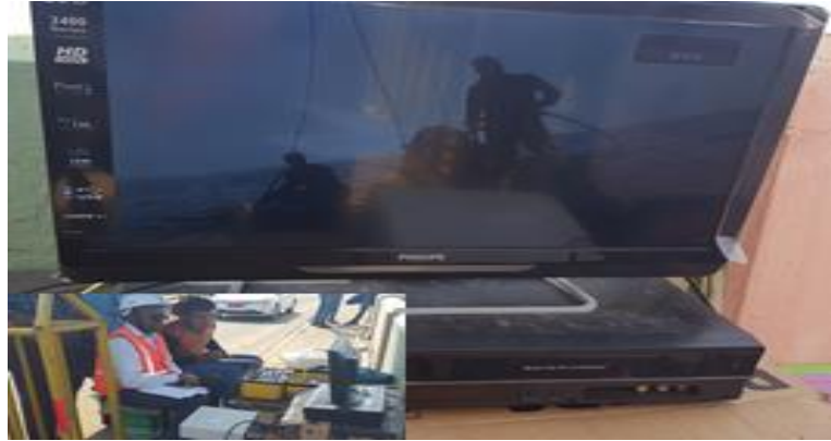
ROV for sluice emergency gate groove underwater repair works at Panchet dam, DVC
