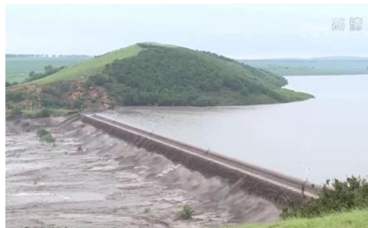
Xinfu dam (China) failure by overtopping (July 2021)
