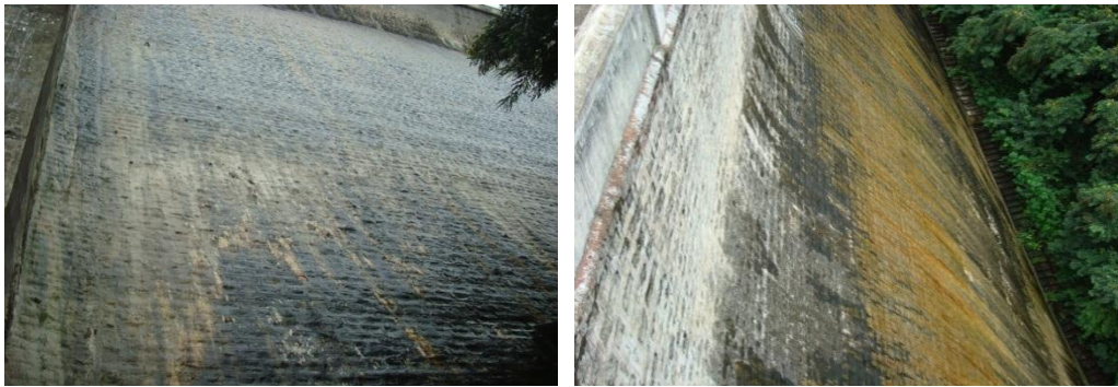
Figure 5. Heavy seepage on left flank.
