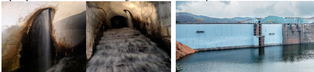
Figure 9. Leakage in vertical shaft of drainage gallery at left. At right, geomembrane lined on the upstream face of the dam as of June 2019.
