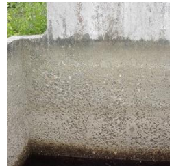
Picture 3: Typical example of soft chemical attack in an irrigation canal
