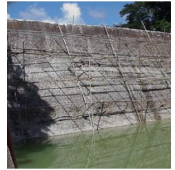
Picture 2: Typical example of erosion by abrasion in a spillway of a small dam.
