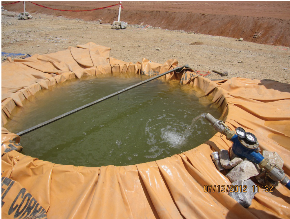
Photograph 4 : Filling density test excavation to determine volume using the water replacement method.
