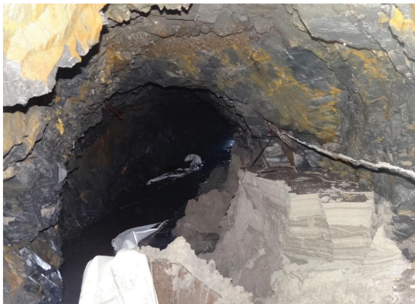
Figure 7 : Silt deposited in exploratory drift of Power House during flood event of 2013
