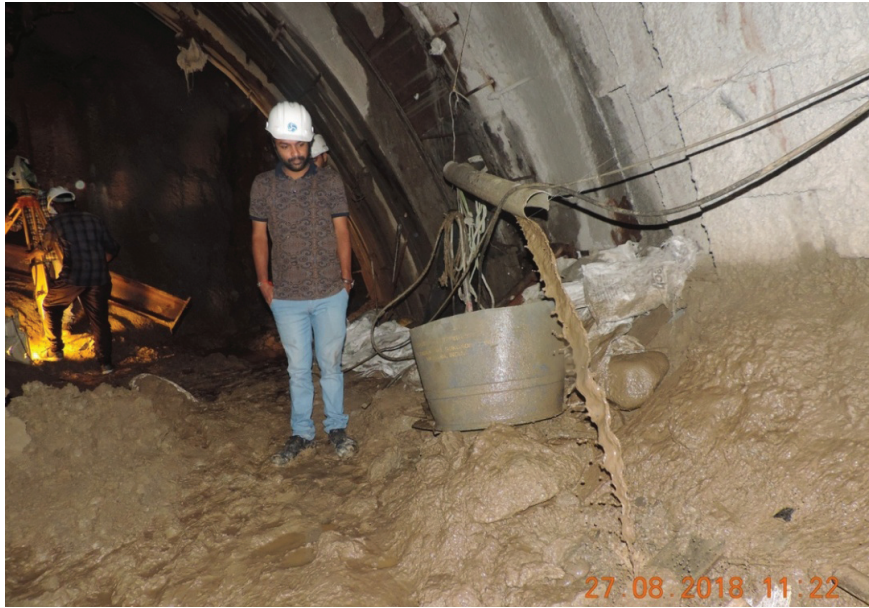
Figure 5 : Gushing of water with silt from right side at RD 41.5m of TBM entry Adit.
