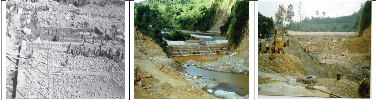
Fig. 2 : Pictures of U/S coffer dam foundation colgrouting, under construction and completed view
