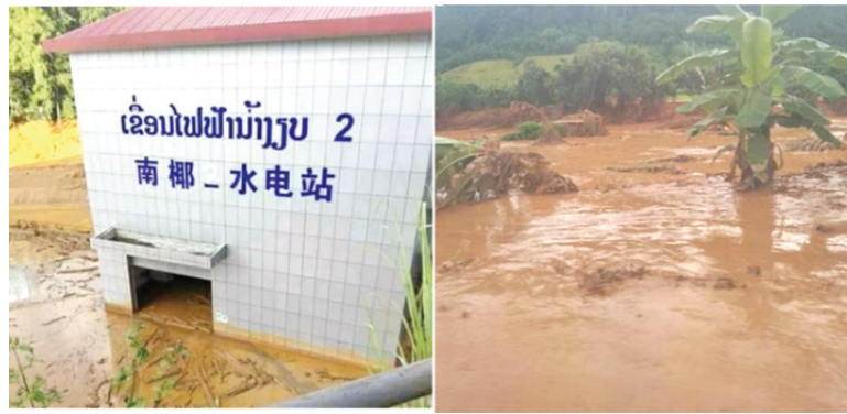
Figure 4 : Damage on powerhouse of NNP2 and agricultural land
