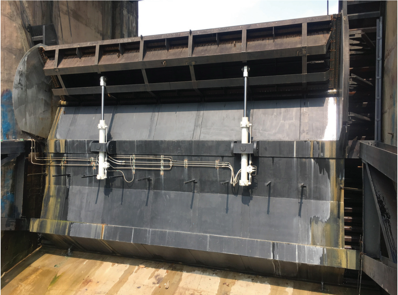
D/S VIEW OF NEW FLAP TYPE RADIAL GATE NO. 12
