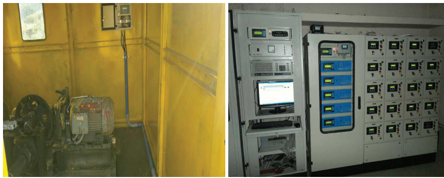
Fig. 5 : SCADA based gate control panel set-up
