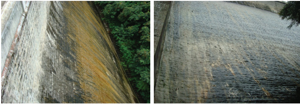
Figure 5 : Heavy seepage on left flank.
