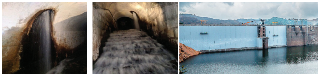
Figure 9 : Leakage in vertical shaft of drainage gallery at left. At right, geomembrane lined on the upstream face of the dam as of June 2019.
