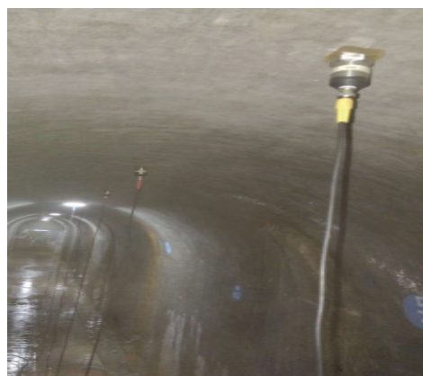
Figure 9 : Receivers –@ceiling of gallery
