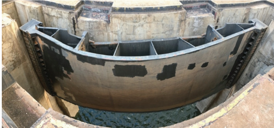
Figure 3 : Downstream face of one of the four elements of the stoplog (the photo is distorted).
