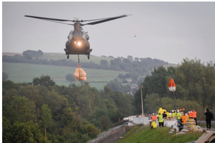
Figure 6 : Scour hole infilling
