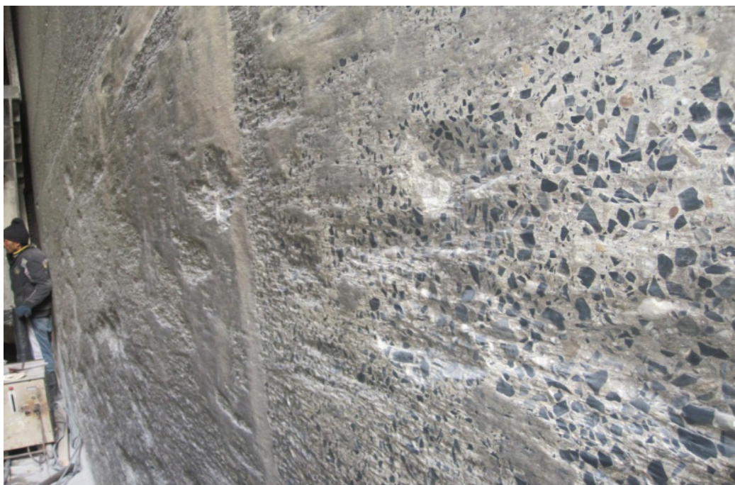
Figure 2 : Erosion in Pier of Dhauliganga Spillway before repair with cementitious mortar(R4)
