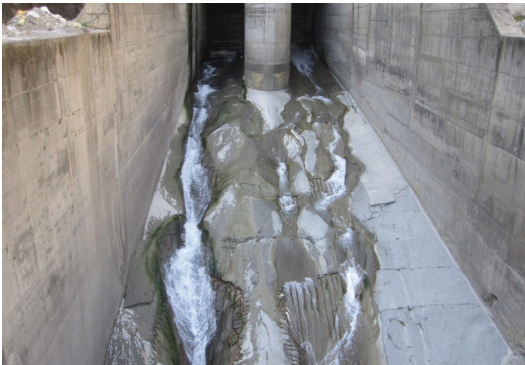
Figure 1 : Erosion in Glacis of Dhauliganaga Dam Spillway before providing steel liners
