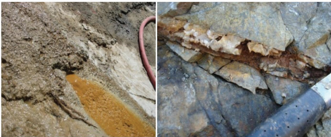
Figure 2 : Wash-out of clay filling joints by pressure washing (MGCE, 2016).
