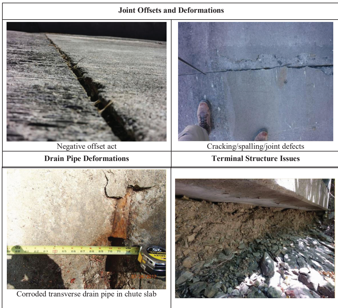
Figure 2 : Example of Spillway Deformations
