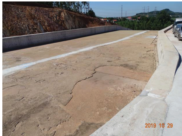
Figure 7.2 : Khe Che Dam: the existing spillway has been widened (the white line shows the side wall of the original spillway)
