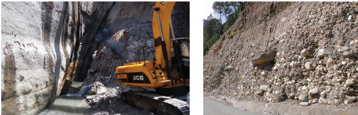
Figure 3 : Abrasion of spillway due to sediment in Maneri Bhali-I (left) and side slopes at the landslide areas near the reservoir, showing the outcrop of alluvial deposits
