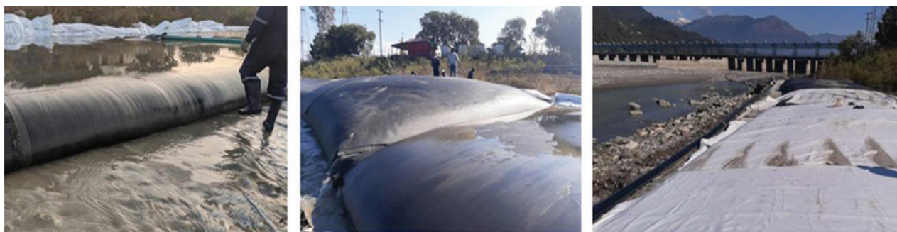
Figure 4 : Bank protection using geotubes downstream of Dakpatthar barrage: an example of reuse of dredged sediment from the reservoir (Omer et al., 2020)
