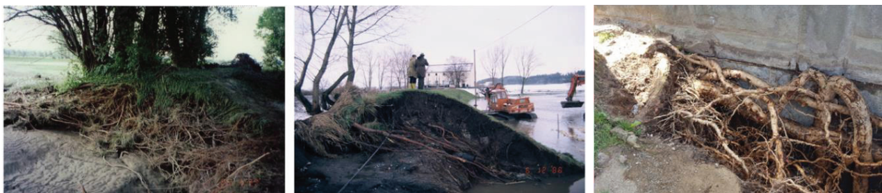
Figure 9 : Rooted levees at the River Ammer (left) (Source: WWA Weilheim) and River Danube (middle) (Source: LfW BY) and excavated roots of a poplar at a flood protection wall in Düsseldorf (right)
