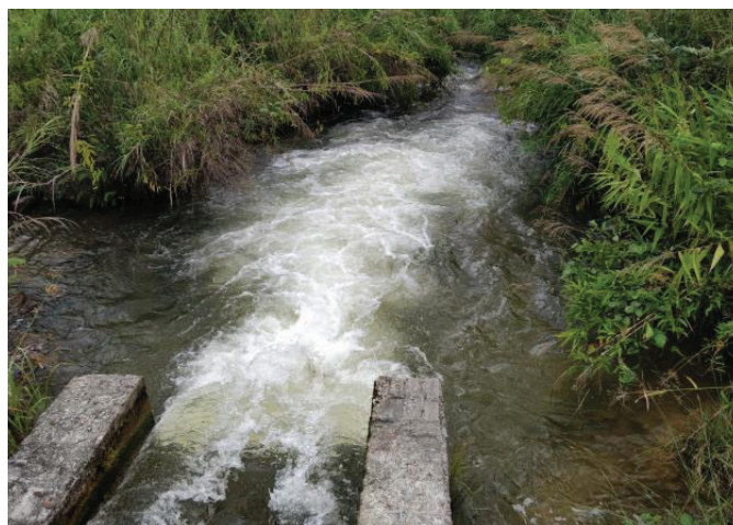
Fig. 1 : Leakage at the measuring weir
