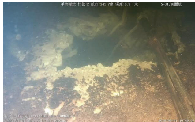
Fig. 4 : Underwater high-definition photography of the leakage hole on No. 38# concrete slab
