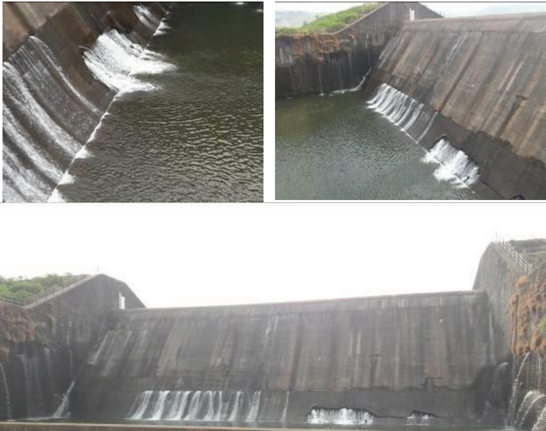
Fig. 1, 2 & 3 : Seepage observed through the spillway and cavities on the glacis concrete
