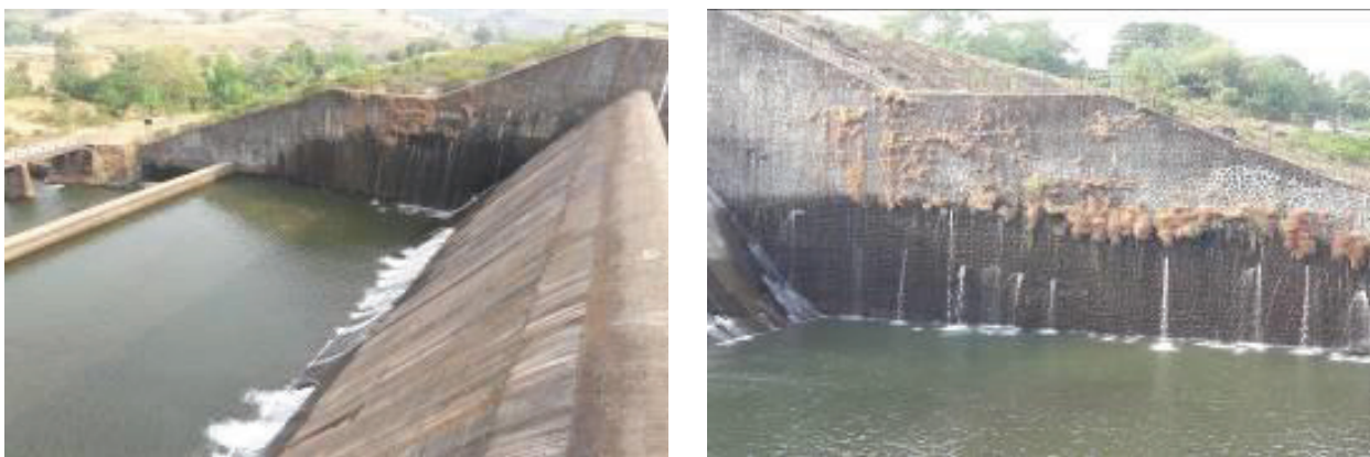
Fig. 4 & 5 : View of seepage observed in right and left flanks of Domihira dam.
