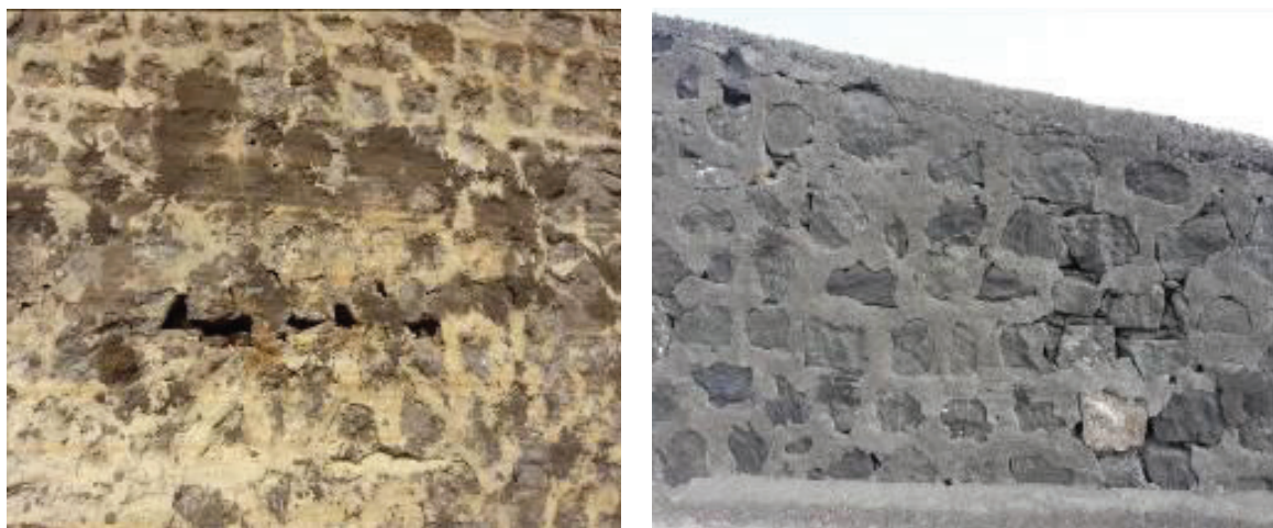
Fig. 6 & 7 : U/s portion of Domihira dam showing cavities in spillway portions and flank walls
