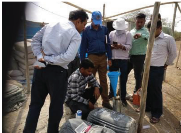
Fig. 11 : Testing of Marsh cone flow value in Domihira dam site before grouting
