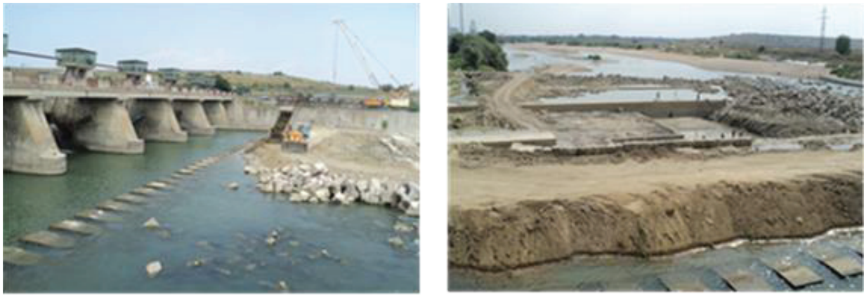
Figure 6 : Construction site after the flood in April 2013.
