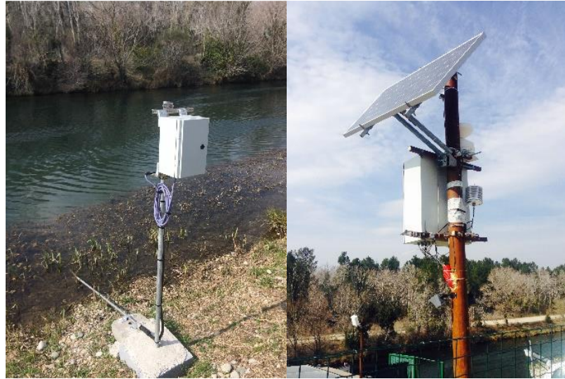
Figure 3. THM Logger on the downside of the embankment (left) Solar system and metrological sensor (right)
