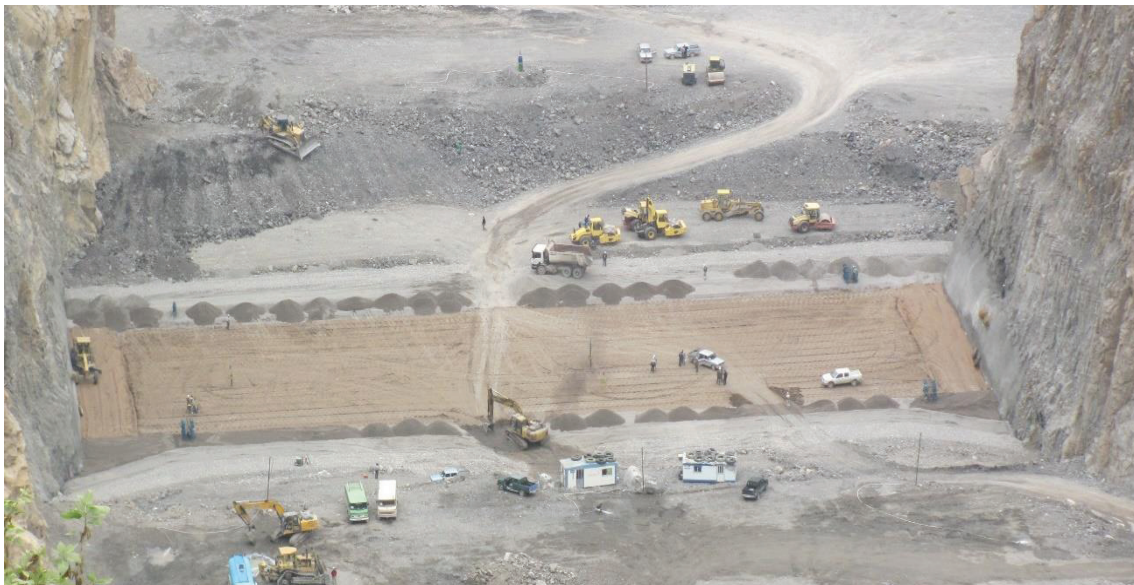
Figure 2 : View of core, 5 m wide plastic contact clay zone at the abutments, 5 m thick fine sand filter widened to 10 m at the downstream contact with the abutment, 5m thick coarse sand filter, 5 m thick transition zone, and rockfill (view from downstream).
