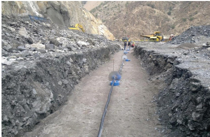
Figure 5 : Installation of horizontal extensometers in dam body.
