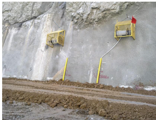
Figure 4 : View of 5 m wide plastic contact clay zone at the abutment, treatment of rock surface in the core and filter zones by shotcrete and slip measuring devices (TDR) installed on abutment.
