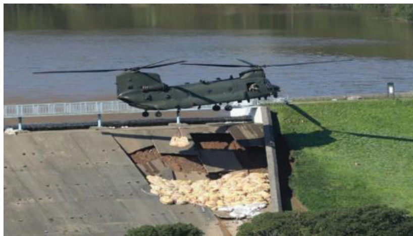
Picture 4 – The Failure at Whaley Bridge
