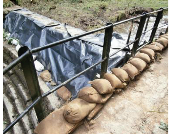
Picture 15 : Temporary Inlet Weir
