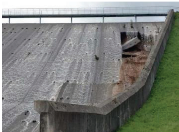
Picture 7 – Initial Failure on the 1 August 2019
