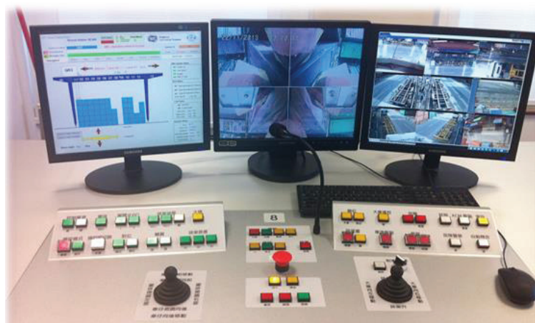
Fig. 2 : Automated centralized monitoring system
