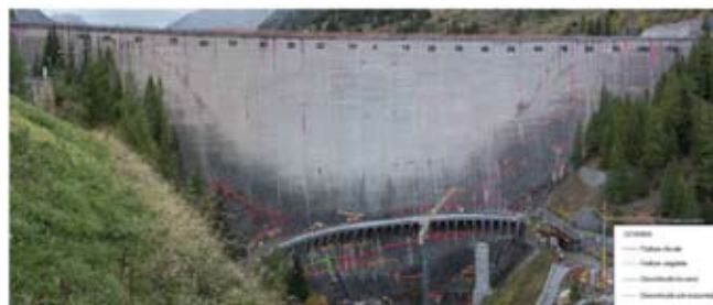
Fig. 2 : Cracking of the downstream face of Beaugard Arch Dam
