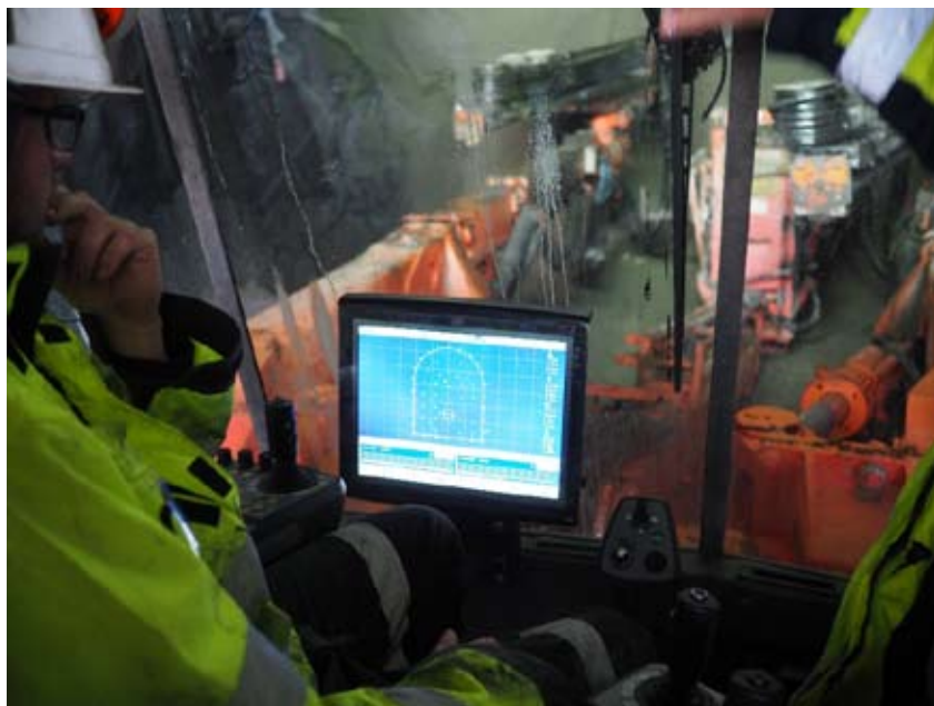
Figure 3 : Borehole contours based on the BIM-model shown on a display in a tunnel rig. Example from the new Mjåvatn dam and water tunnel in Norway.
