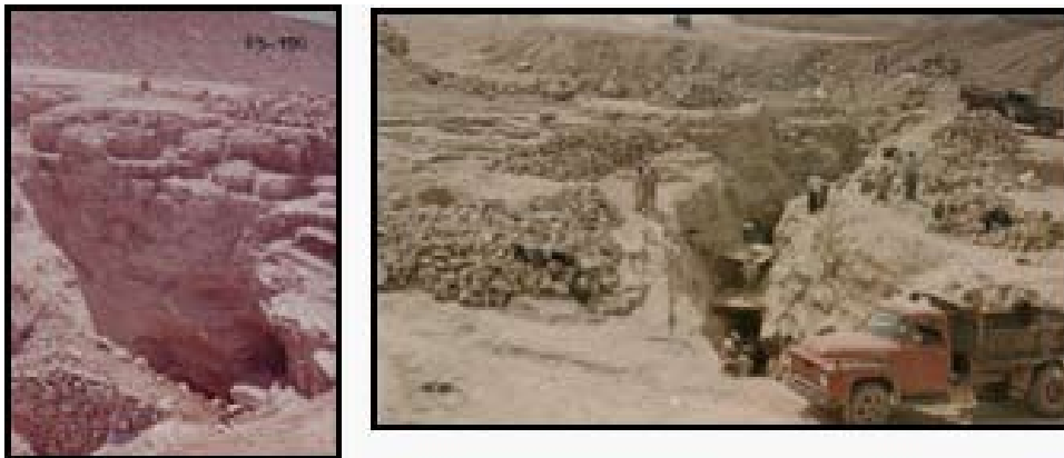
Figure 6 : Photographs of Cavities Encountered at Station 6+460 During Construction
