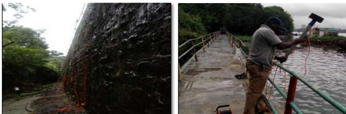
Figure 9 : Locations of Geophones at the downstream face and upstream face of the Powai dam
