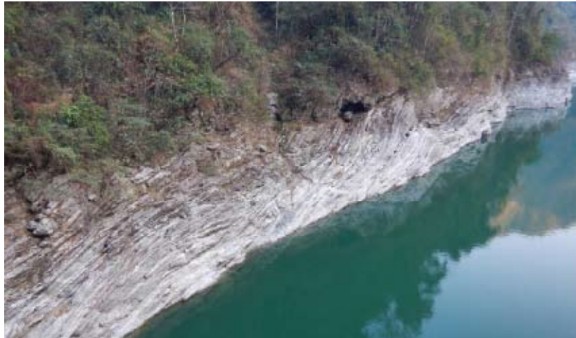
Fig 2 : Foliation joints with highly varying dip directions exposed towards left bank upstream of dam axis.
