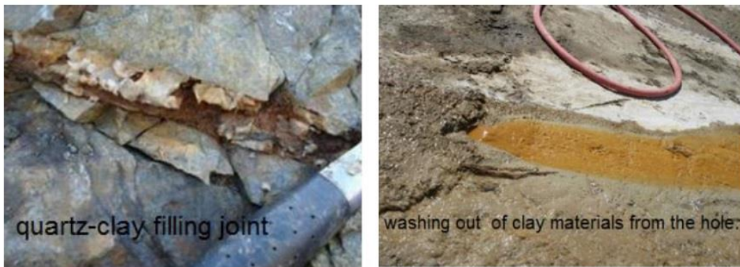
Figure 8. Left: quartz-clay filled joint, Right: pressure washing of clay filling
