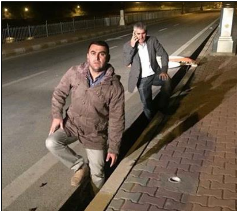
Figure 3 Visual inspection just after the earthquake.
