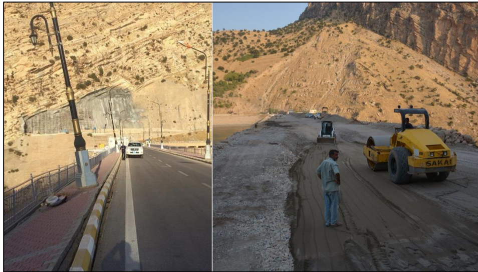
Figure 11: The crest of the dam before and after removing the damaged parts.
